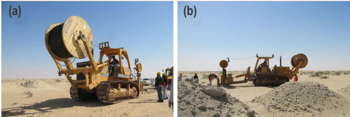
Figure 13—Cable ploughing machines deploying continuous cables in shallow trenches as a method of automated placement of DAS seismic cables for surface seismic.
